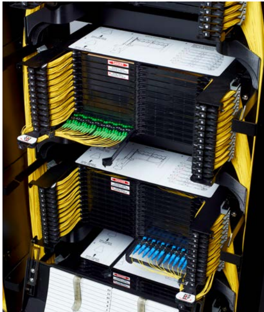
Access Trays with (2) LC 12 and (2) SC 6 Adapter Packs Installed
