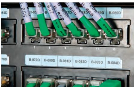
Patch Panel Labels
