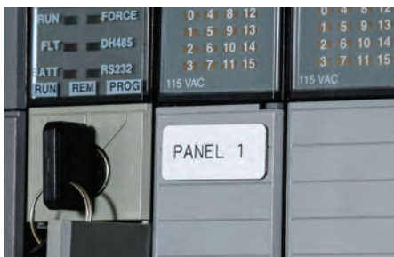
Control Panel Labels
